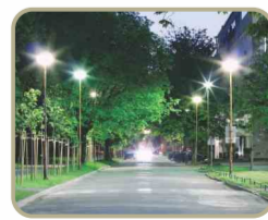
SOLAR STREET LIGHT
